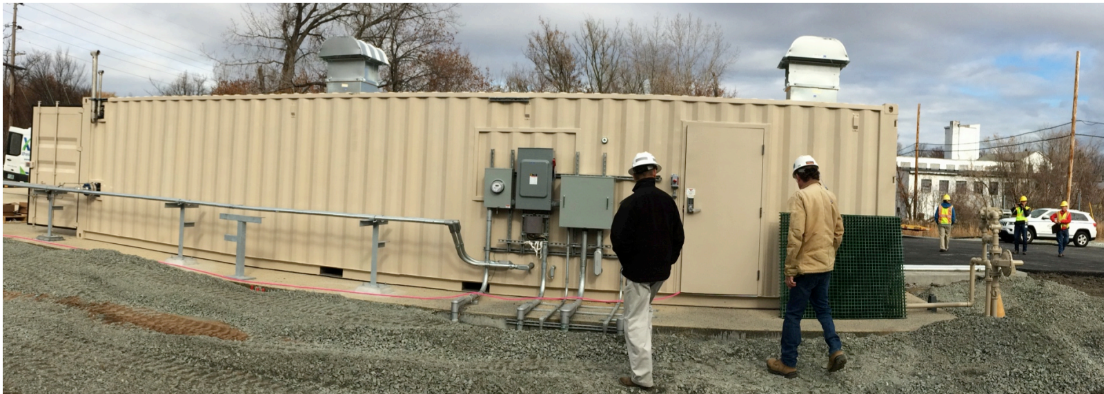
NYSEG Facility (New York State Electric and Gas) in Mechanicville, NY
