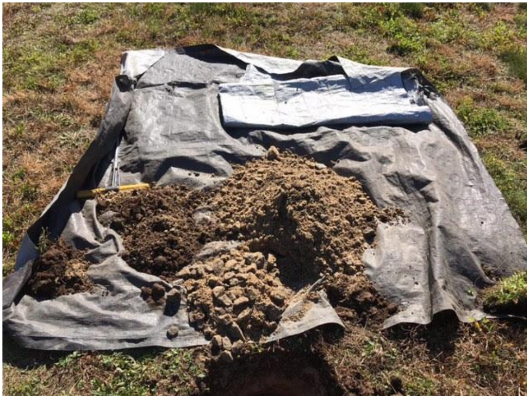
FIELD A - Observation hole #3 sand and stone
