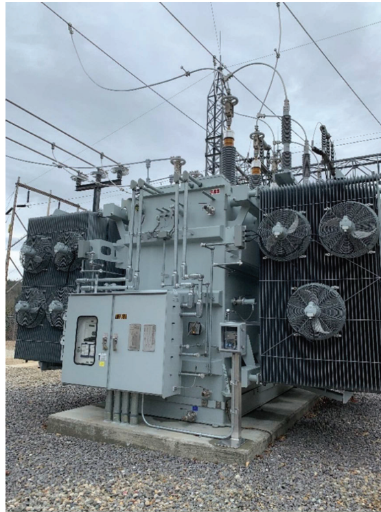
Figure 5-45. New 62.5 MVA Transformer at Pemigewasset Substation
