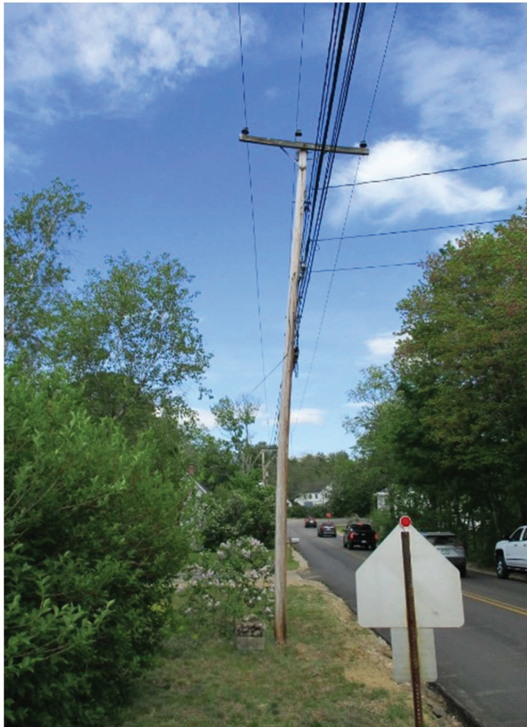
Figure 4-5. Structurally Overloaded Eversource Class 4 Wood Distribution Pole
