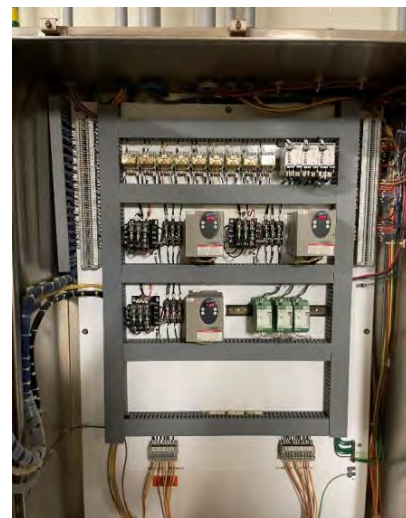
This photograph from PWW's Pre-Treatment Chemical Area depicts the interior of an electrical cabinet housing three chemical pump variable frequency drives.
