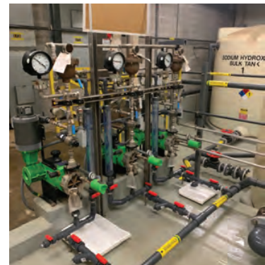
Existing PWW sodium hydroxide chemical feed pumps. New chemical feed pumps could be replaced in the existing facility, or located in a new structure nearby.
