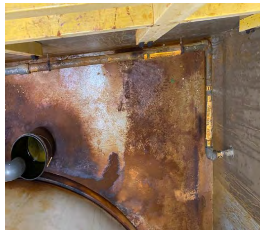
Figure 3-5. Caustic Soda Piping in the Ferric Chloride Bulk Tank Storage Area
