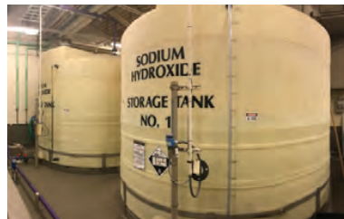
Sebago Lake Water Treatment Facility Chemical Storage Tanks CIP Development Portland Water District, Portland, ME
