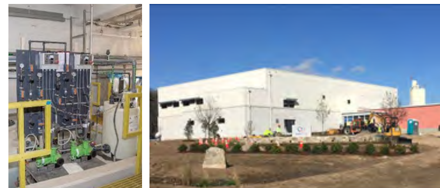
Phosphate Chemical System
