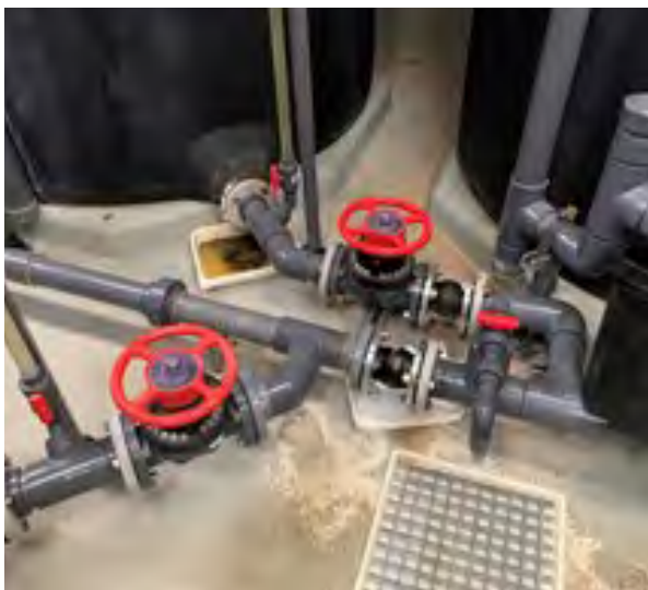
Leaking outlet flange from Hypochlorite IMFO bulk tank
