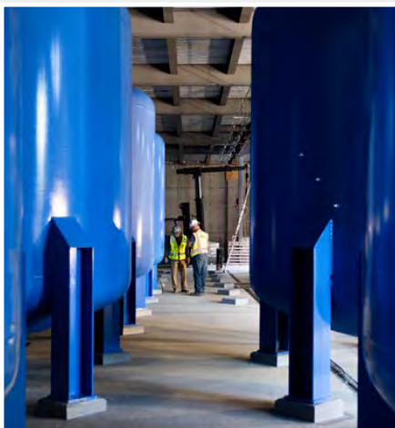
Topsham Treatment Facility.
