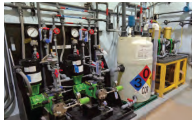
Revitalization of Existing Water Supplies City of White Plains, White Plains, NY
