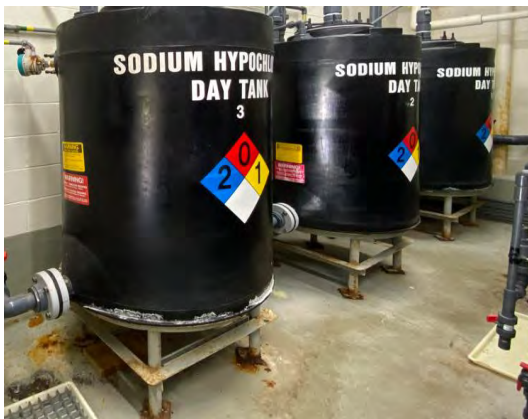
Figure 3-2. Deterioration of Sodium Hypochlorite Day Tank Metal Stands
