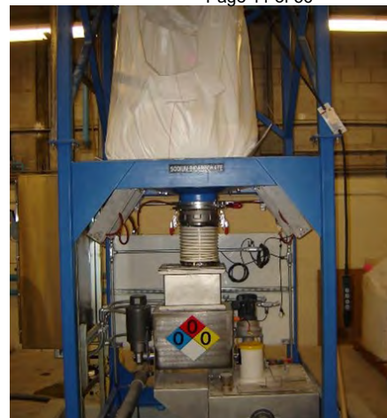
New Bicarbonate Feed System
