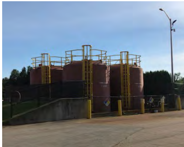
Philip J. Holton Purification Plant, liquid ferric sulfate exterior bulk storage tanks
