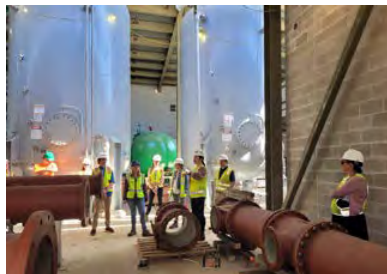
Ji Im addresses colleagues, Contractor, and MWW staff at recent site visit, educating the audience of the benefits of this new facility.
