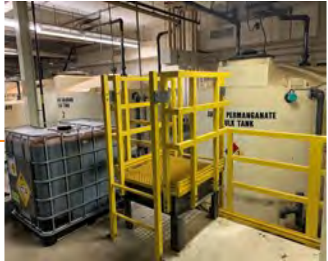
Permanganate Tank Re purposed as Ferric Chloride #4
