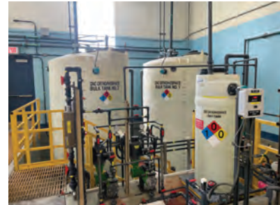
■ Post-Chemicals - Zinc Orthophosphate
