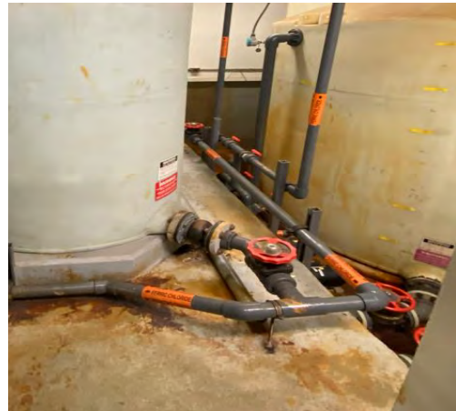
Figure 3-4. Lack of Fall Protection Between the Day Tank Area and the Depressed Bulk Tank Area
