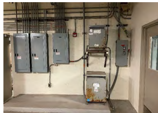
This photograph from PWW's Pre-Treatment Chemical Area depicts electrical panels and transformers exhibiting age and corrosion.
