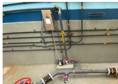
Figure 3-6. Transfer Pump Disconnect Partly Inside the Secondary Containment Area
