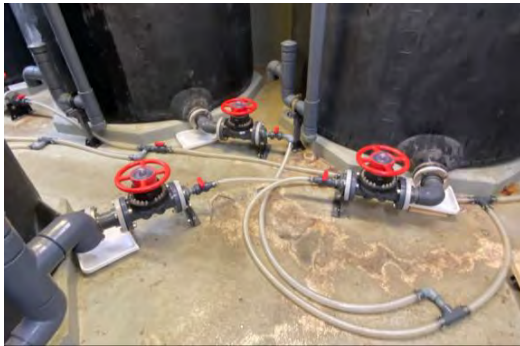
Figure 3-1. Floor Deterioration in Sodium Hypochlorite Bulk Storage Room
